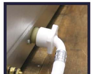
Water Inlet for Steam Injector
